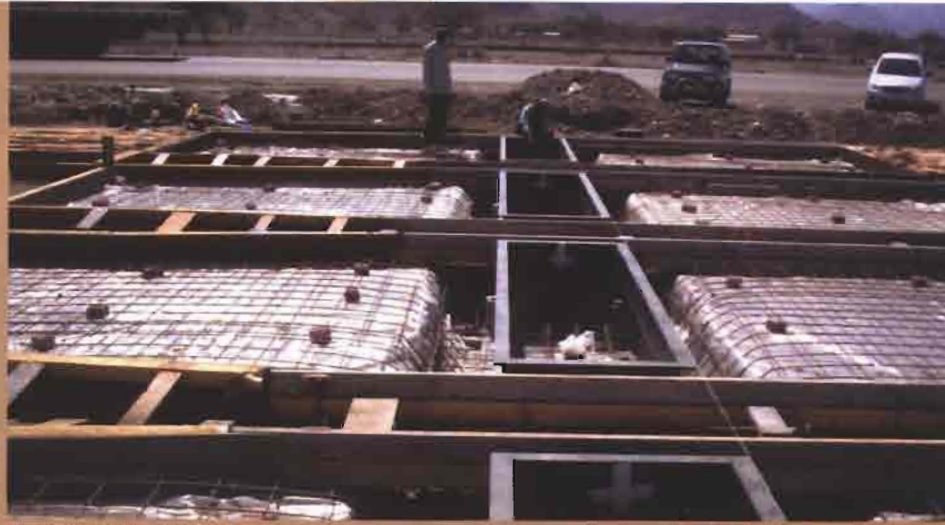
Installing four of 30 lanes of Supaweighs, weighing over 9,000 vehicles a day in the U.A.E.
